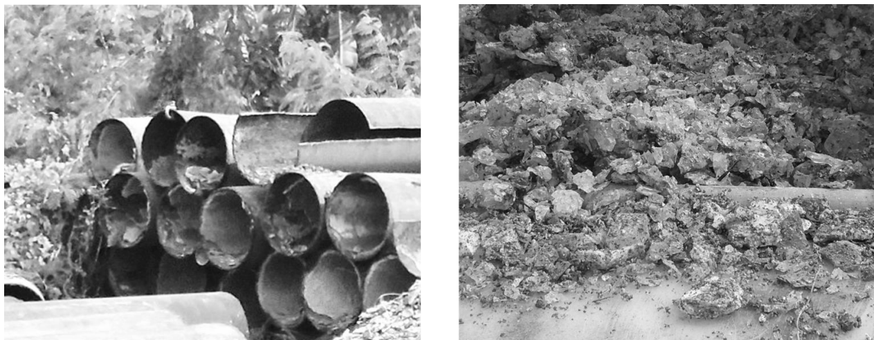
Figure 1. Photo of the pipe scale in the geothermal plant.
